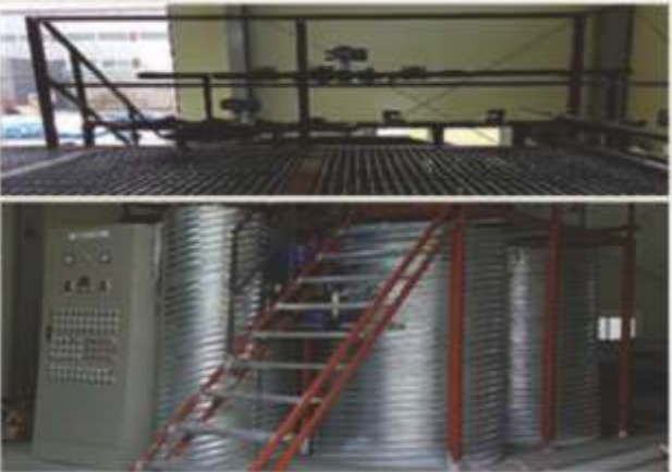
(50m 3 /d, 100KWh/d) PKG CSBR Interior (BOD 5 <10, TN<20, TP<1.0 mg/l)
